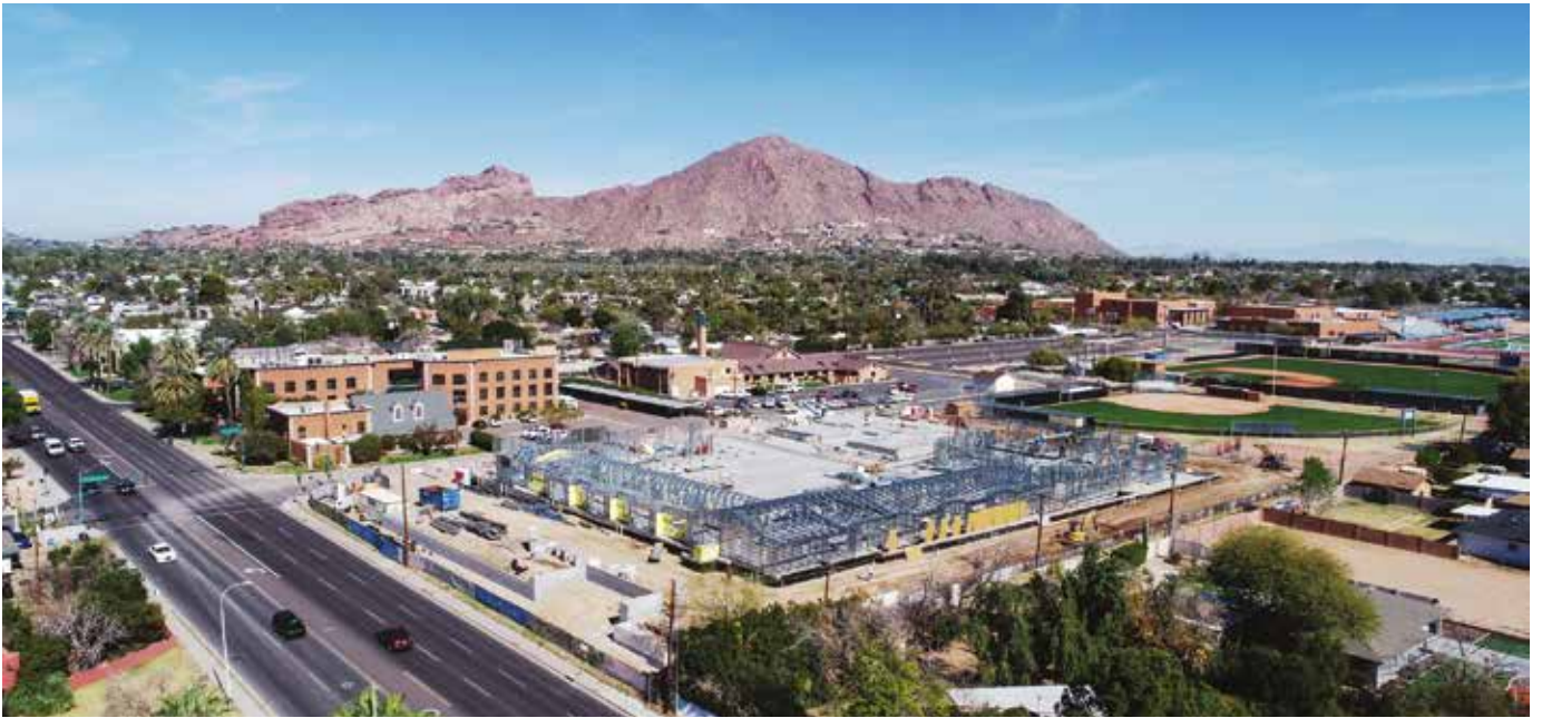
The Dementia Care and Education Campus is under construction near 44th Street and Indian School Road.
